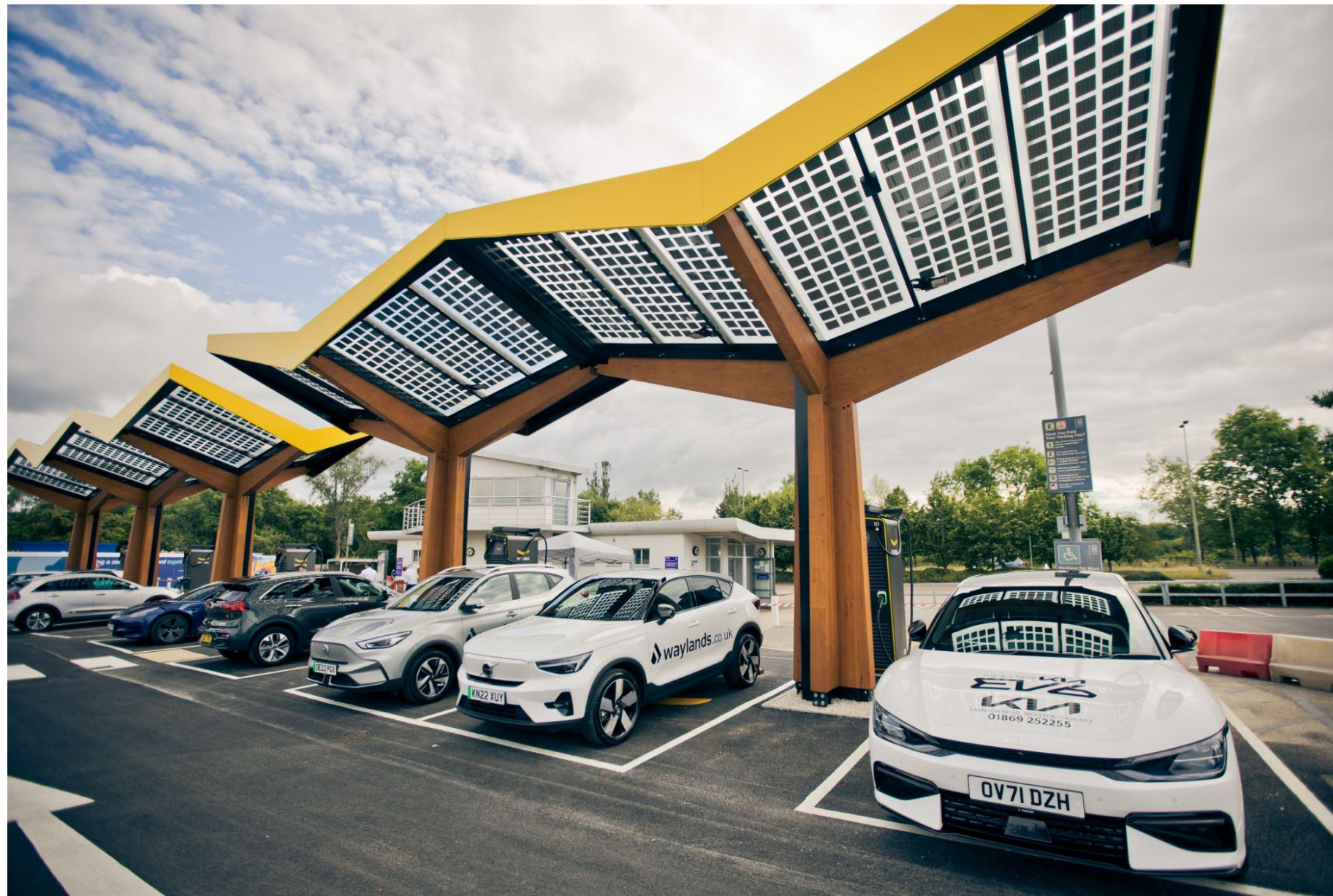
Oxford Redbridge (the UK) 10 x 300 kW chargers
